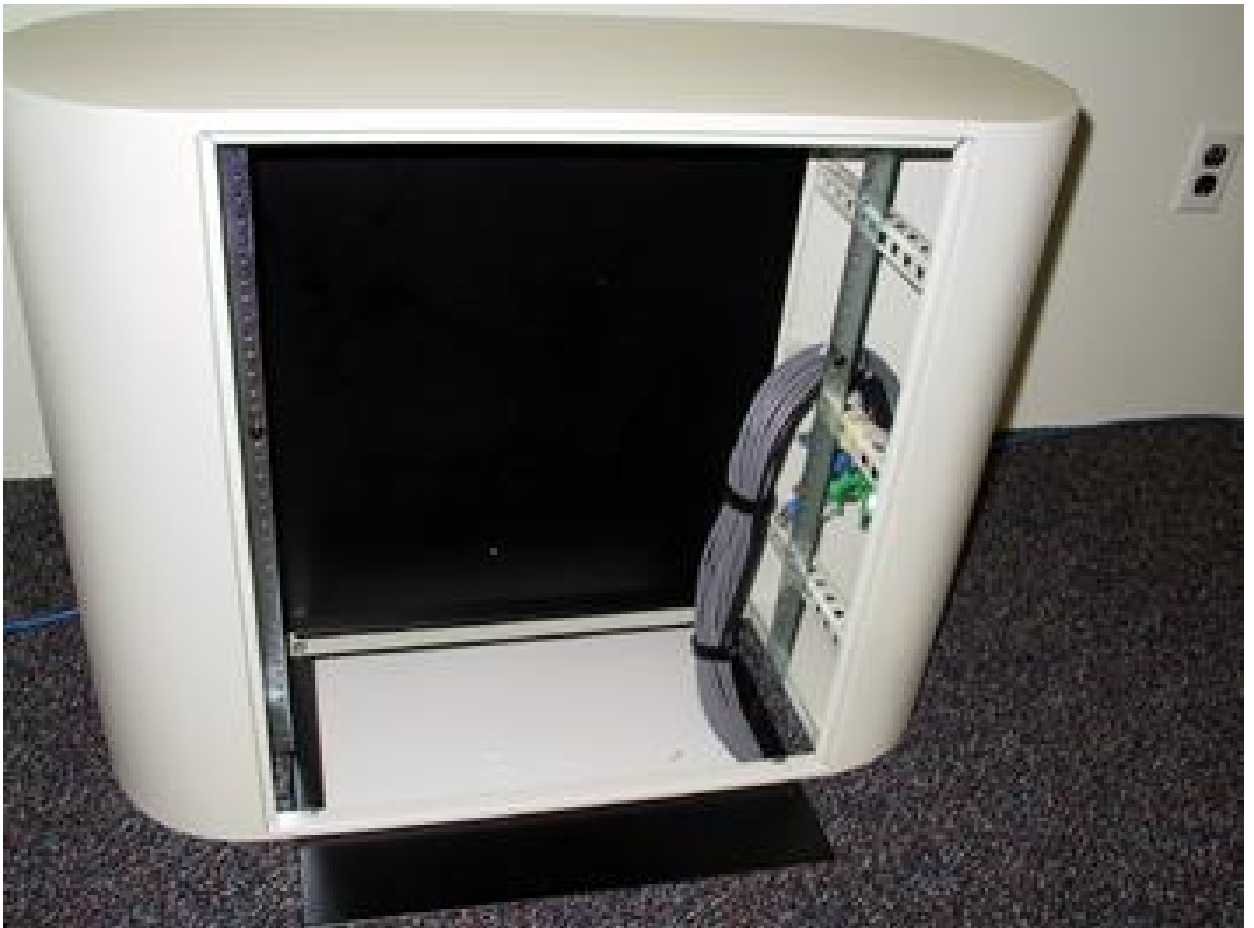
LDS with Data Cables fed through
