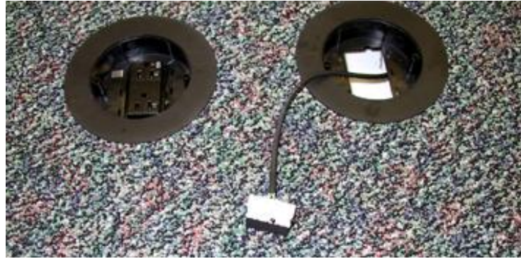
Picture 10-23 Mod-Edge end of Data Cable through Powerport
