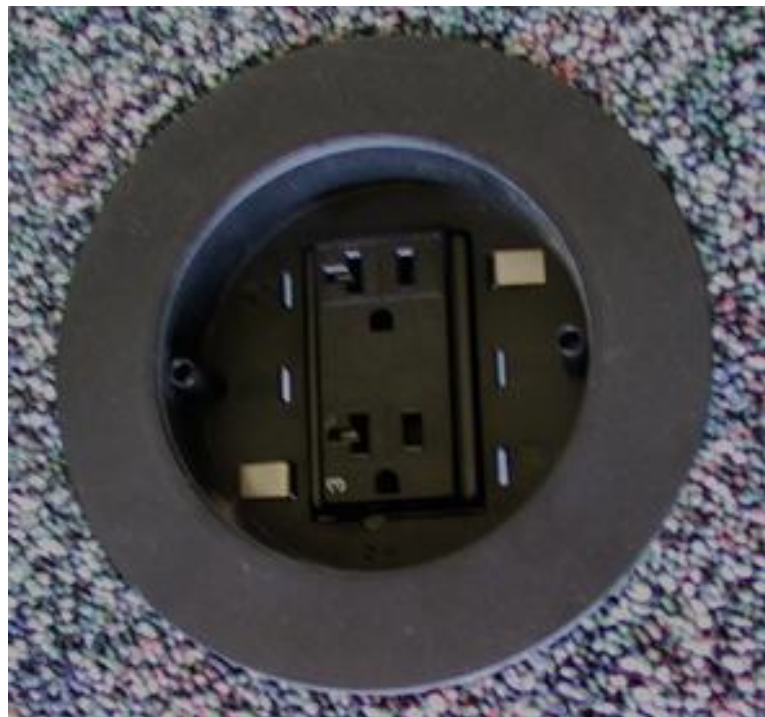
Completely Installed Electrical Outlet ( Top View )
